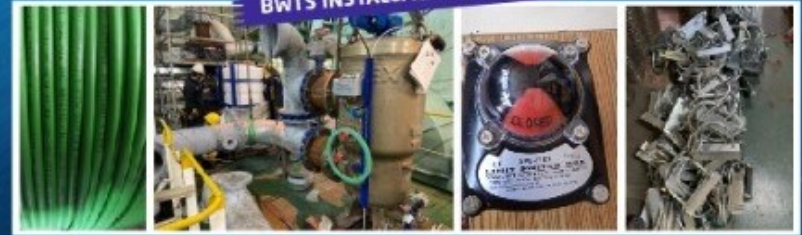
BWTS INSTALLMENT & PARTS
